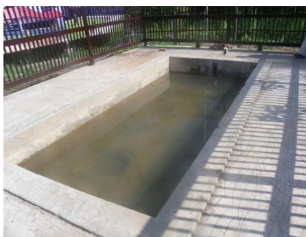
Holding tank No.2
