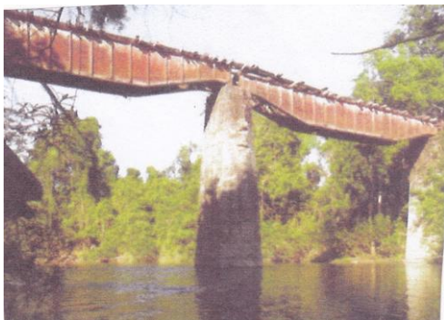
Bridge post war
