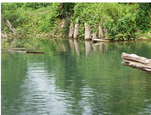
Remains of the large timber trestle bridge adjacent to the steel bridge
