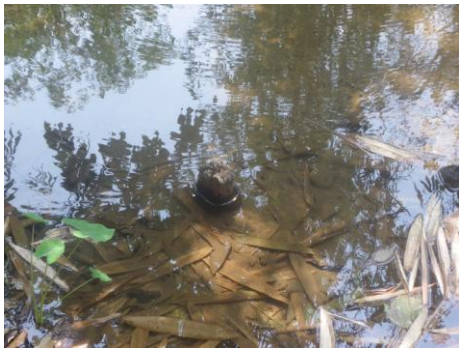
Remains of timber piles at third river crossing
